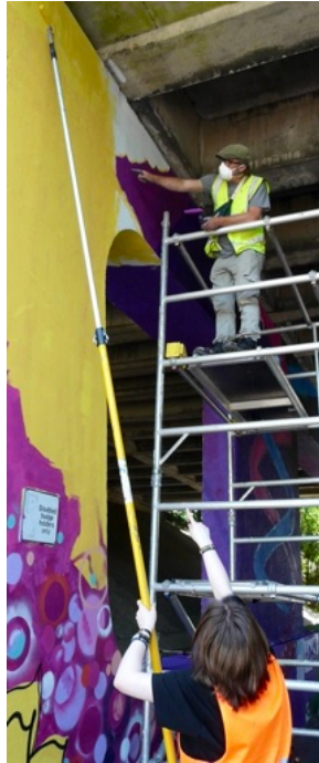
Work in Progress on the underpass mural: Alex Singleton working with a TOA pupil. Read more about this project in the next issue.
